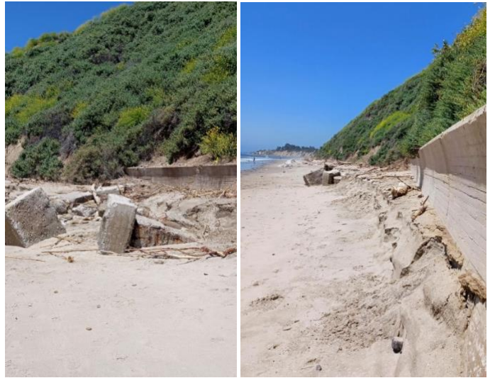
The sand level is 5 ft down or more in places, revealing concrete blocks previously buried under the sand. At the end of the wall, there is a concrete “bench” for sitting.
