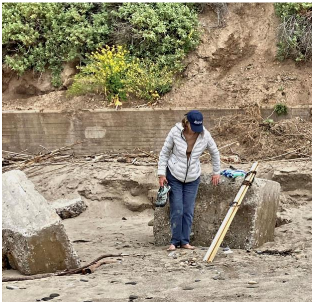
Lower sand levels reveal hidden concrete fallen from the cliff above Bates. See Page 2.
